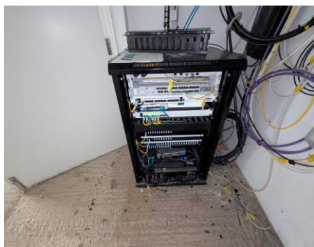
PHOTOGRAPH 16 VIEW OF EXISTING ELEVATE PRIMARY CABINET
