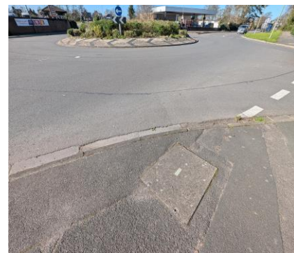
PHOTOGRAPH 3 EXISTING VIRGIN MEDIA CHAMBER IN FOOTWAY ON THE CAUSEWAY NEAR TO ESTATE ACCESS ROAD
