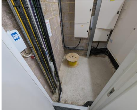
PHOTOGRAPH 26 TYPICAL INTERNAL VIEW OF EAST TENANT RISER
