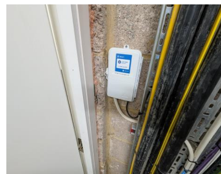
PHOTOGRAPH 18 TYPICAL VIEW OF ELEVATE FIBRE BFP WITHIN EAST TENANT RISER
