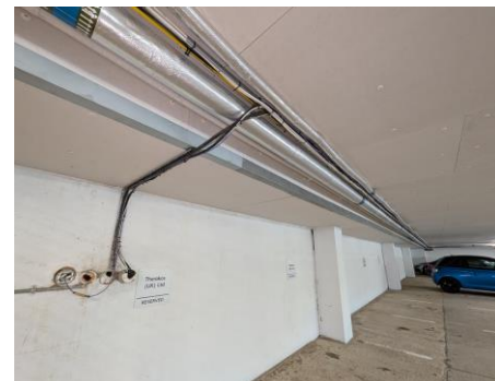
PHOTOGRAPH 15 VIEW OF CABLE ROUTE BACK TO INTAKE CUPBOARD AND LOCATION OF VODAFONE BFP
