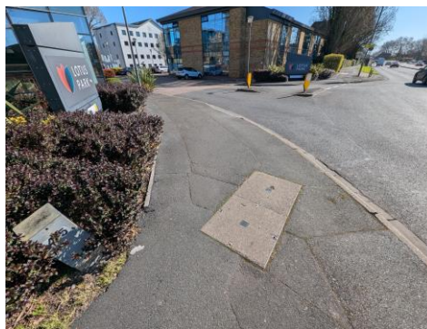
PHOTOGRAPH 2 EXISTING VODAFONE CHAMBER IN FOOTWAY ON THE CAUSEWAY NEAR TO ESTATE ACCESS ROAD
