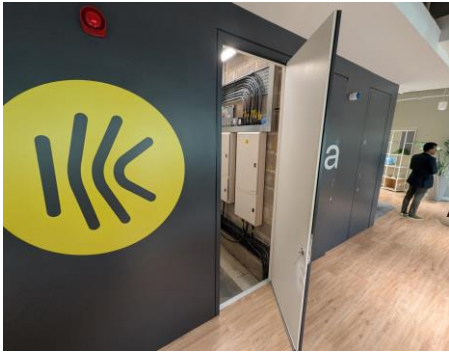
PHOTOGRAPH 22 TYPICAL EXTERNAL VIEW OF WEST TENANT RISER
