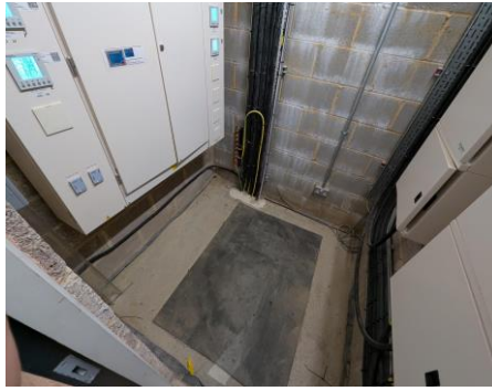
PHOTOGRAPH 23 TYPICAL INTERNAL VIEW OF WEST TENANT RISER
