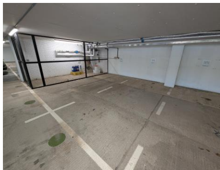
PHOTOGRAPH 13 VIEW OF SECONDARY INTAKE WITHIN BASEMENT CAR PARK
